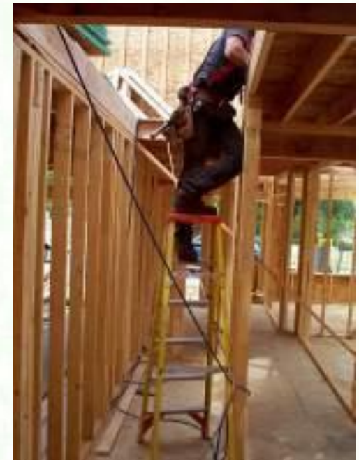
Unsafe access with stepladder
